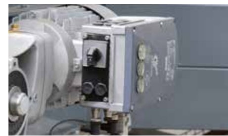
Switches and buttons are located directly on the drive units and enable direct starting, stopping or mode changes.
